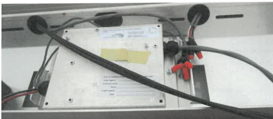
Figure 20. ECM with solar, LED and battery wires
